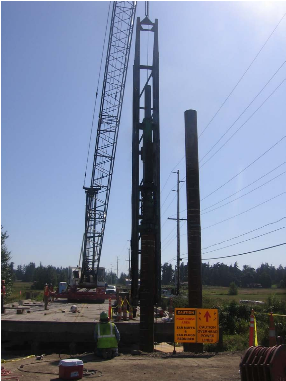
The piles for the new bridge are driven to 90 feet below ground and filled with reinforcing steel and concrete
