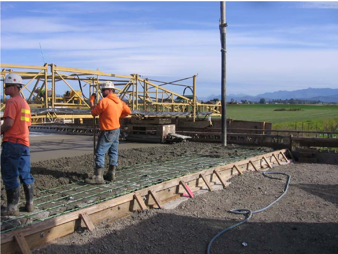
Casting the new reinforced concrete bridge deck on top of the girders
