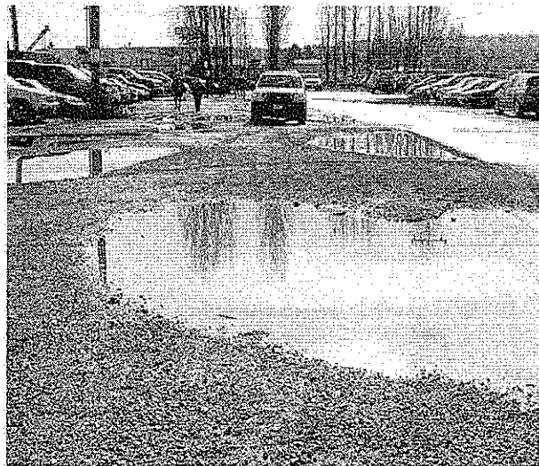
There's no stormwater system in parts of Seattle's Georgetown neighborhood, so stormwater either puddles on the street or runs into the Duwamish River.
